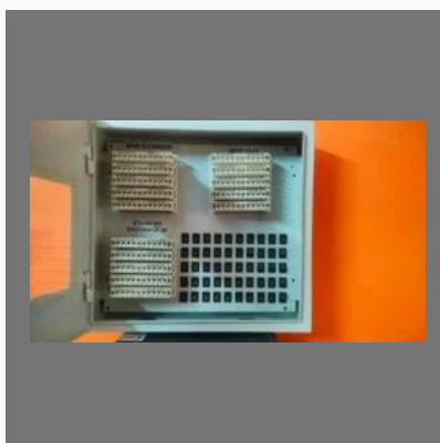
Change Over Switch For Standby EPABX
