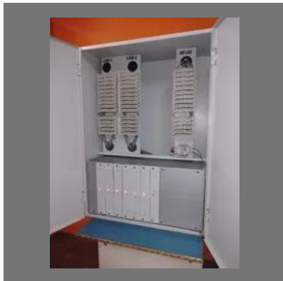
Switching Stand By EPABX System
