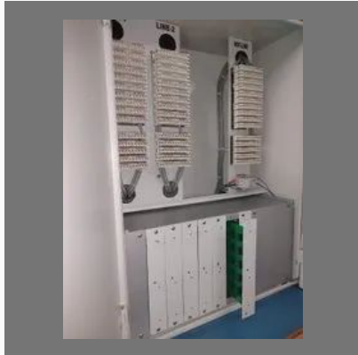
Change Over Switch Stand By EPABX System
